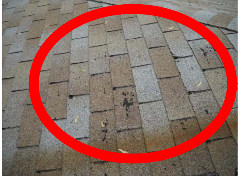
The main roof surface and the flat roof area have signs of worn out shingles and loose seams on the flat roof. Recommend replacement in the next 2-3 years.
