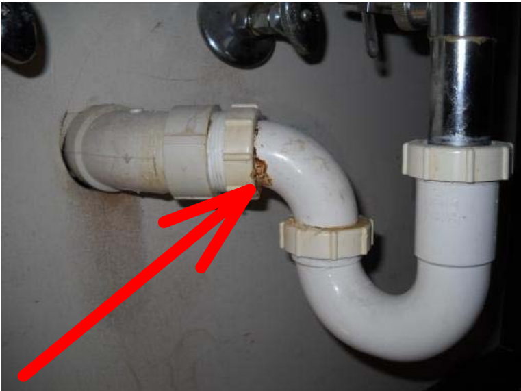
The right side sink drain connection has an active water drip from the rear drain pipe in the upper hall bathroom. Recommend repair.
