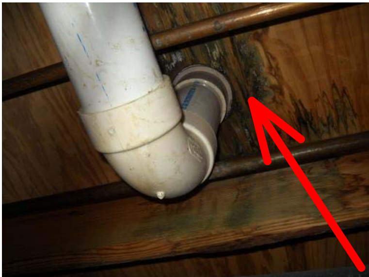
The plywood subflooring is moisture damaged under the lower hall bathroom toilet. Recommend replacement of the subflooring when the toilet repairs are performed.
