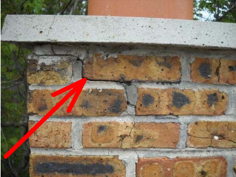
Bricks have broken or popped surfaces with cracking mortar joints. Recommend repairs be made by a qualified masonry contractor.
