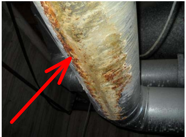
The heating return duct behind the furnace is rusted through on the bottom side from the toilet leak. Recommend having a qualified heating contractor replace this section of the duct work.
