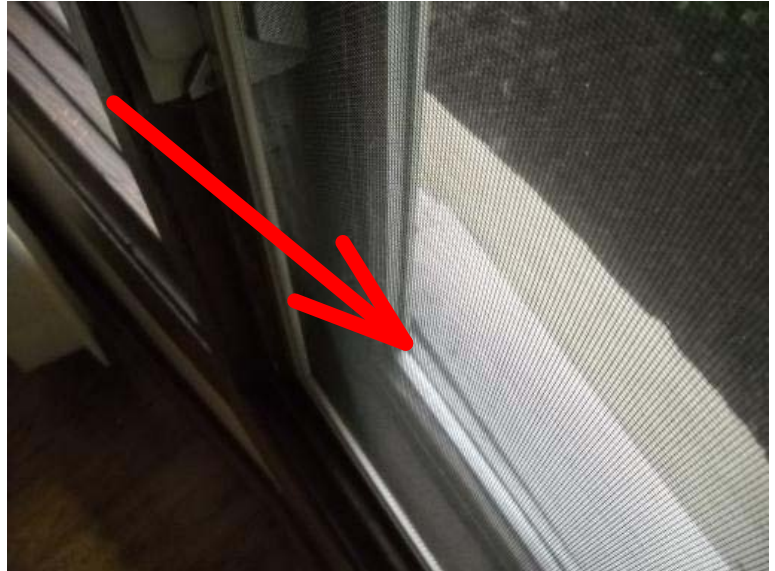
The front living room casement windows bind on the lower exterior window trim and the left window casement is stripped. Recommend repair.
