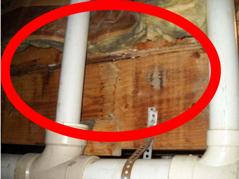
At the basement behind the furnace there are previous water stains from he shower pan in the lower hall bathroom. These stains were dry at the time of the inspection. Recommend monitoring this area for possible leaks and future repairs.
