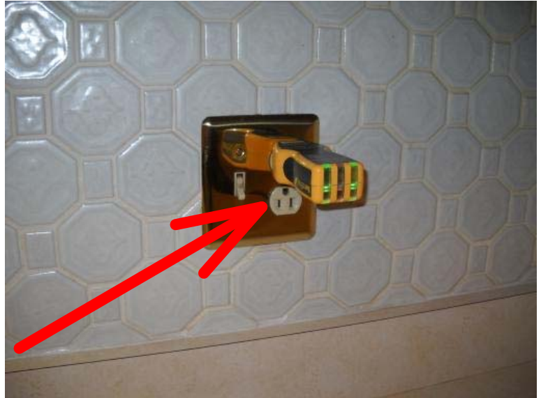
Non-GFCI circuit at the kitchen wall outlets. Recommend a qualified electrician install a GFCI outlets for safety near water.
