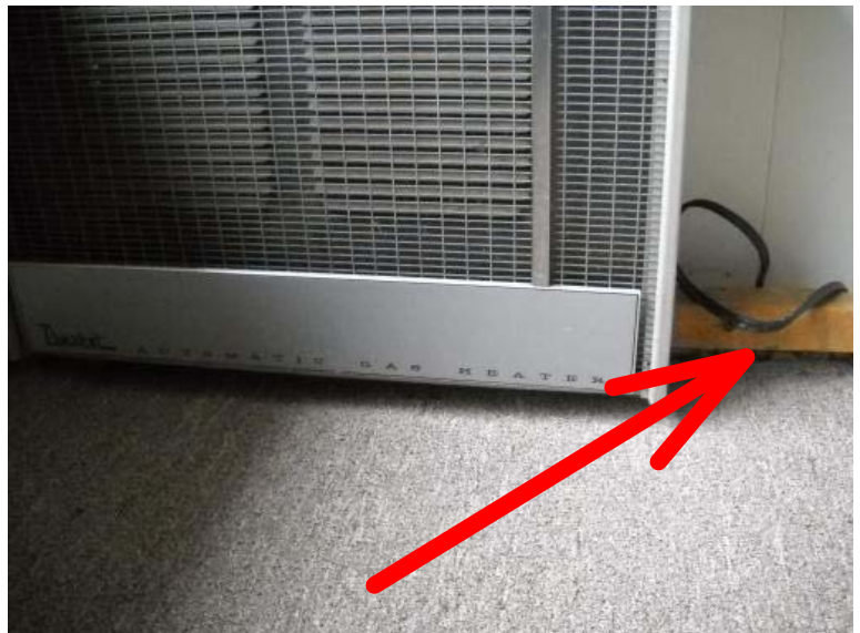
The wall unit heater in the rear sun room has the gas supply turned off and was not able to be function tested. Recommend verifying proper operation prior to closing with the current home owner.
