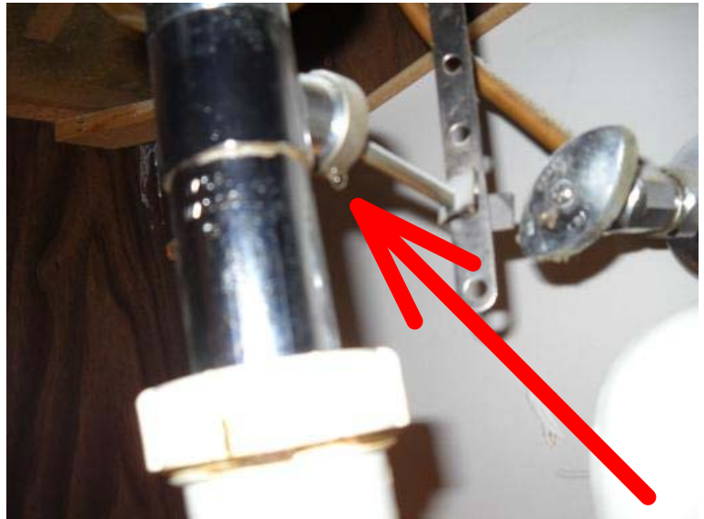
The left sink drain stopper connection under the sink in the upper hall bathroom has an active water drip into the cabinet area. Recommend repair.
