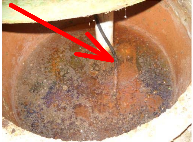
The basement sump pump pit is full of water and the pump will not work when activating the float switch. Recommend evaluation and repair or replacement of the sump pump by a licensed plumber.
