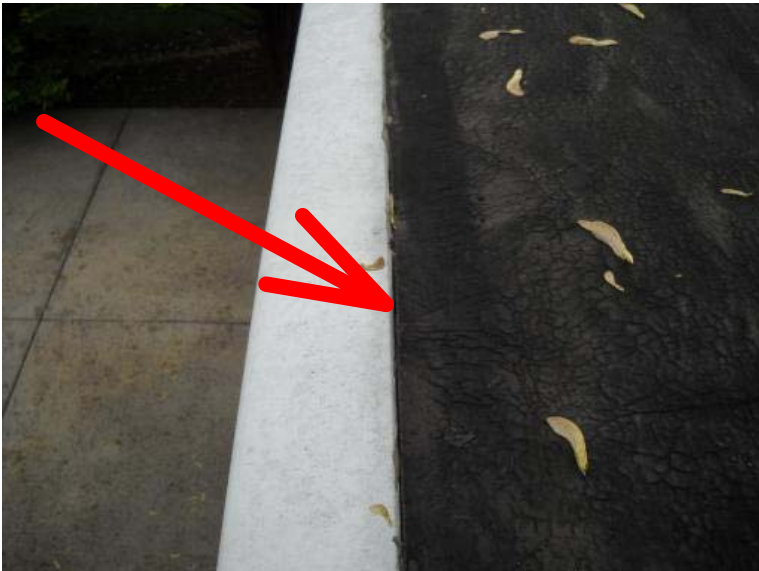
The main roof surface and the flat roof area have signs of worn out shingles and loose seams on the flat roof. Recommend replacement in the next 2-3 years.
