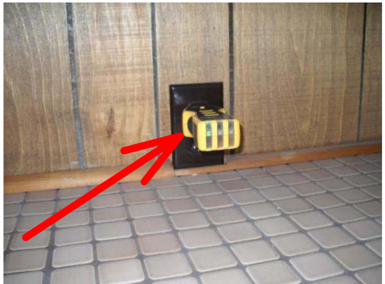
The wall outlet at the left rear corner of the bar area is wired incorrectly with an open ground. Recommend repairs be made by a qualified electrician.
