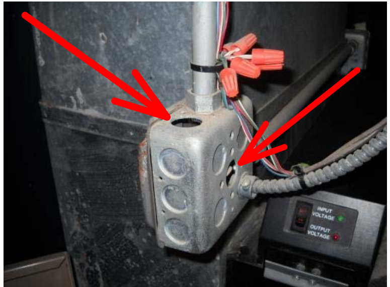
The junction box near the furnace has open knock out holes. All knock outs should be capped for safety.
