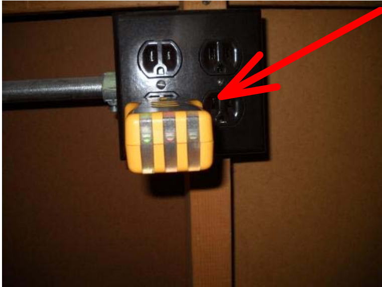
The four bank wall outlets at the bar are wired incorrectly with the hot and neutral wires reversed. Recommend having a qualified electrician properly wire the outlets.
