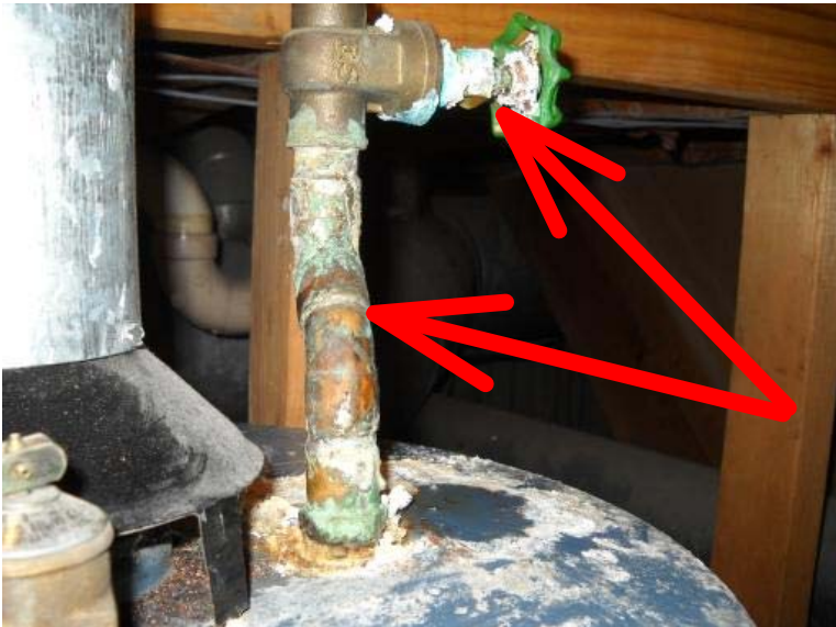
The water shut off valve at the water heater has an active leak and the supply line is corroded. Recommend repair or replacement of the water shut off valve and line by a licensed plumber.
