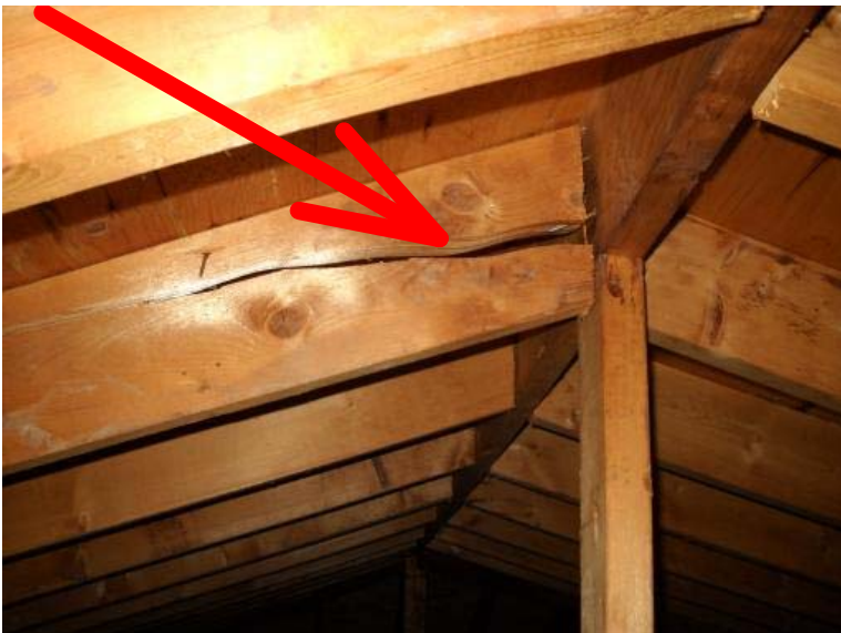
There is a broken roof rafter at the middle front attic area of the laundry room. Recommend having a qualified contractor repair the rafter for proper roof support in this area.
