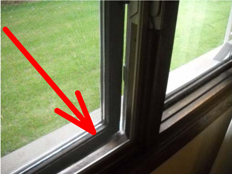
The left window in the dining room will not open properly. It appears the lower sill plate is warped. Recommend repairs be made to the window.
