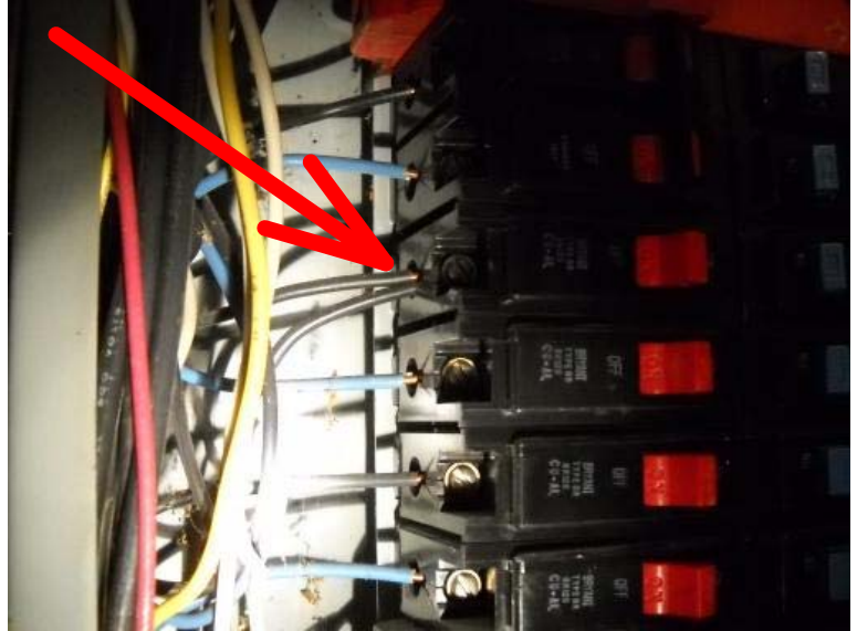
" A double tap, which can result in loose wire connections and possible overheating, was noted. Further evaluation by a qualified electrician is recommended".
