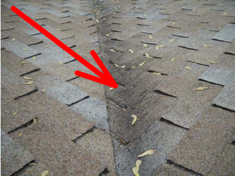
The valleys of the roof are worn with deteriorating shingles. See recommendations under the main roof.
