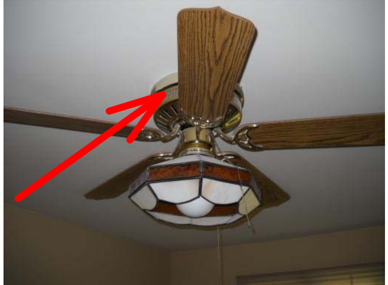
The ceiling fan in the master bedroom is loose at the ceiling mounting. Recommend repairs be made for safety.
