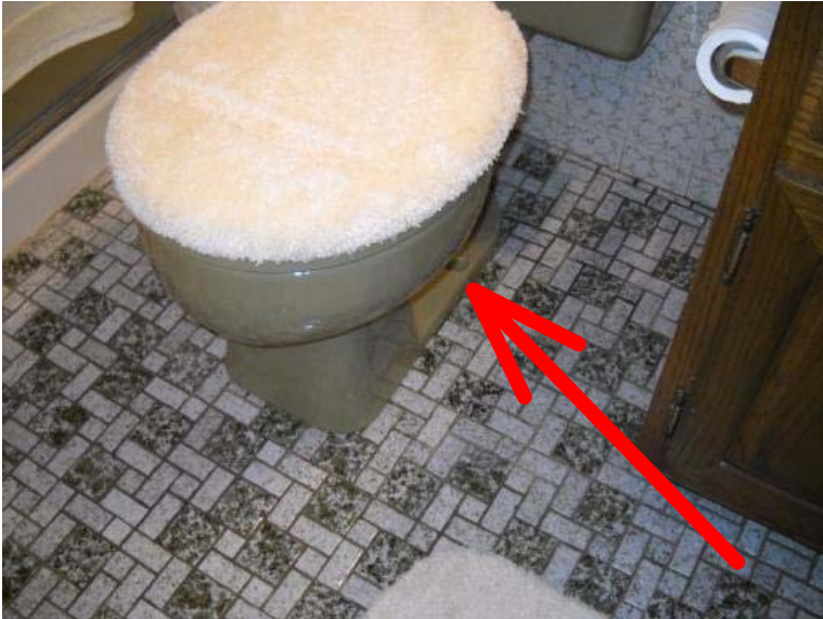
The toilet is loose at the floor mounting in the lower hall bathroom and leaks into the basement behind the furnace. There is subflooring damage at the base of the toilet. Recommend having a licensed plumber evaluate and repair prior to using.
