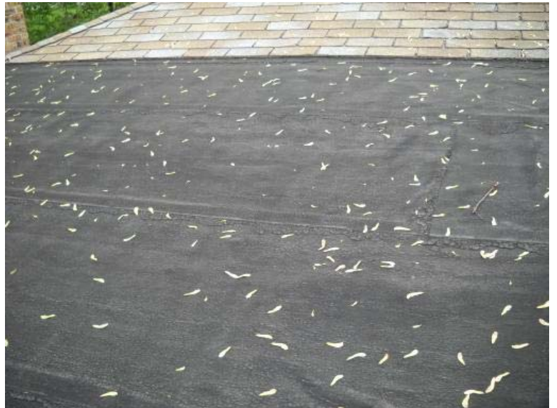
The main roof surface and the flat roof area have signs of worn out shingles and loose seams on the flat roof. Recommend replacement in the next 2-3 years.
