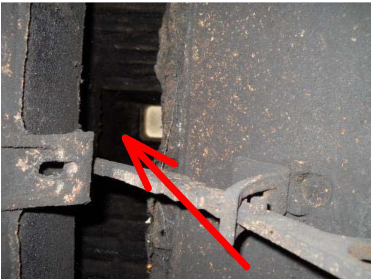
Cleaning of the flue and it's internal components are recommended annually to maintain safety and efficiency of the fireplace.
